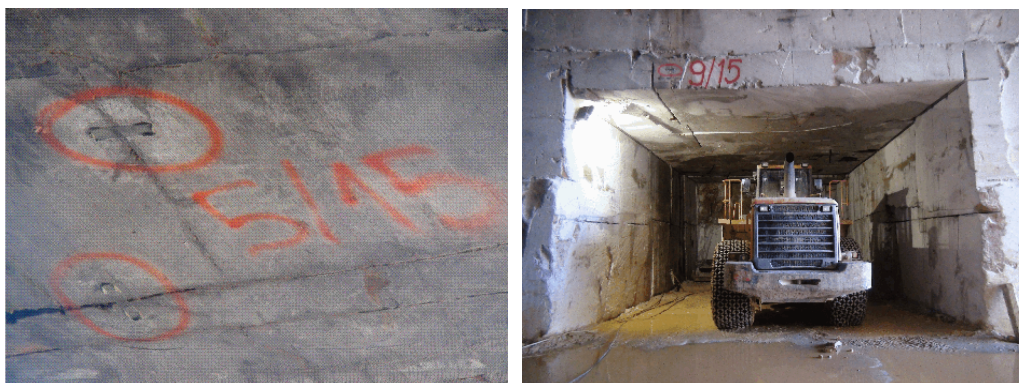
Figure 7.: Visual inspection of open cracks (glass and cement seals) on the ceiling (left) and side of the underground gallery G1 (right).
